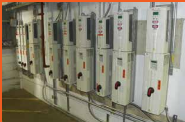
Our Variable Flow Demand Drives use patented algorithms to optimize the total chill water system at Siemens', Roanoke, Virginia plant.
